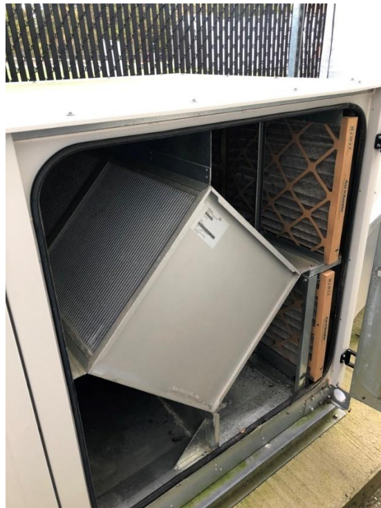
Figure 1: ERV-2 heat exchanger
